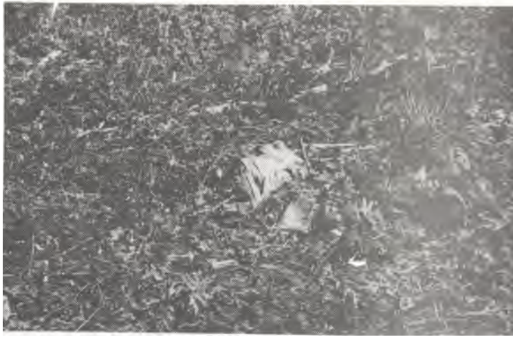
Site prepared for planting. Large stump in center of photograph has been pushed into the ground by the weight of the crusher.
