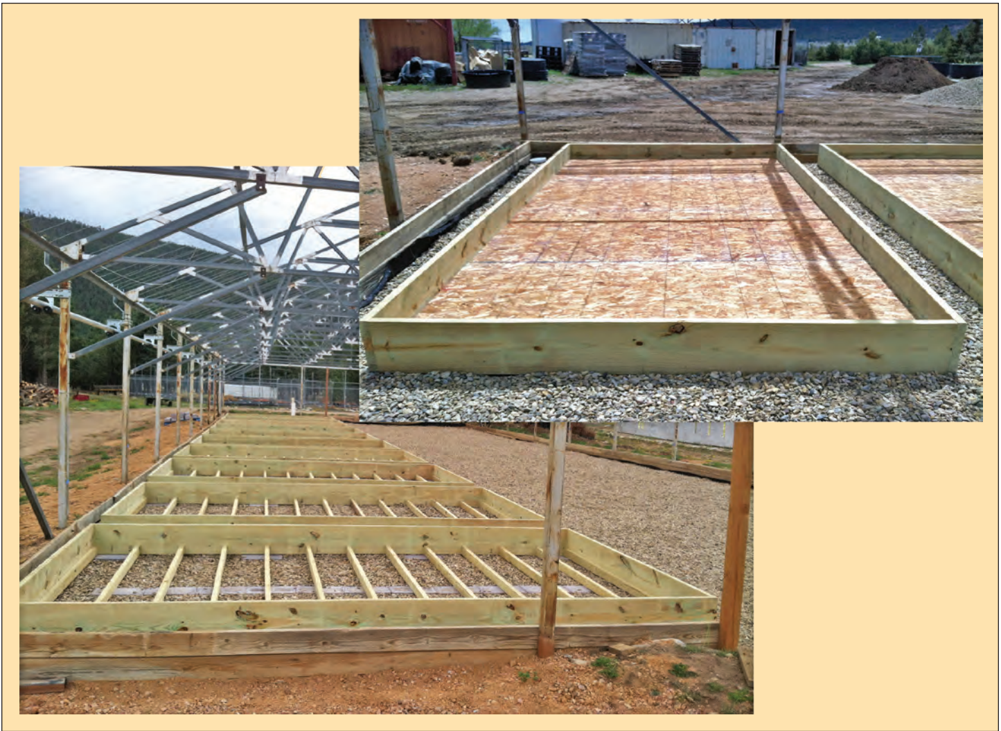
Figure 5. Subirrigation frame and flooring during installation process at the John T. Harrington Forestry Research Center in Mora, NM. (Photo by Tammy Parsons, 2015)
