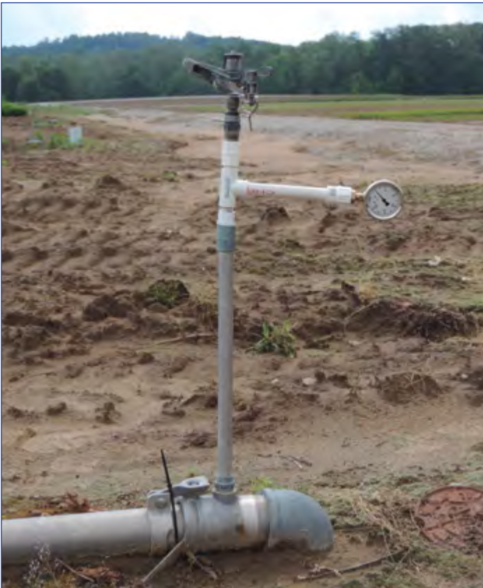
Figure 4. Measuring water pressure with a pressure gauge installed on a riser. (Photo by Ronald Overton 2014)
