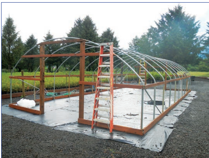
Figure 13. Shade house being constructed at the Oregon Youth Authority Camp Tillamook Work Study Center to use for direct sowing and outdoor natural stratification over the winter. The shade cloth protects seed from bird and rodent predation yet allows for ambient temperatures and rain. (Photo by Kurt Heckerth 2012)
