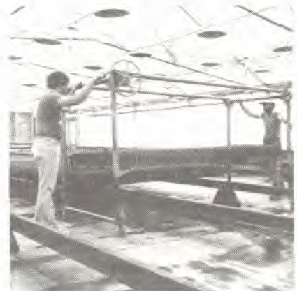
Figure 2—A bunker carrier is used to move bunkers from the headhouse to the greenhouse.
