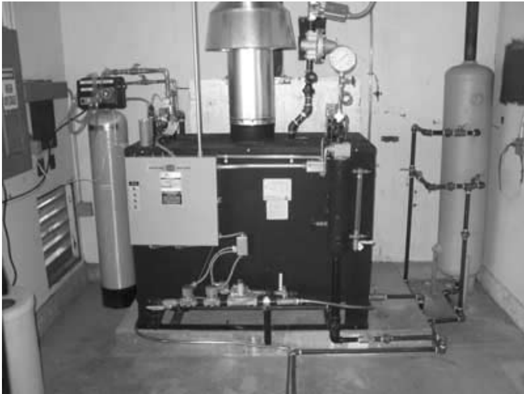
Figure 1 —This propane boiler supplies 160 °F (71 °C) steam to a 24 by 47 by 10 ft (7.3 by 14.3 by 3 m) room used to sterilize used Styrofoam™ containers.
