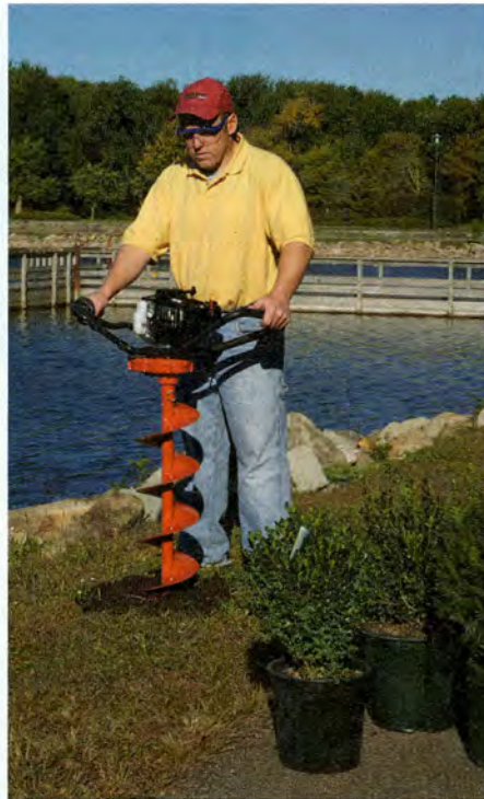
Proper maintenance and operation of hole digging equipment make the job so much easier for landscape professionals.
