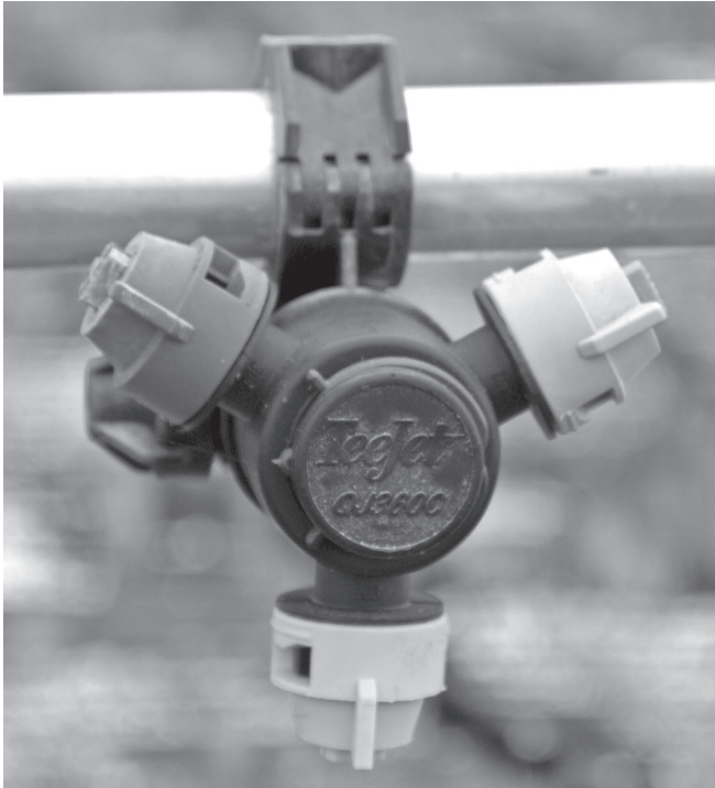
Figure 5 - Irrigation booms can be fitted with special nozzles that allow growers to change from standard irrigation to misting.
