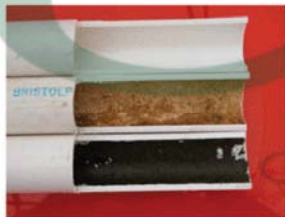
Top: New length of schedule 40 PVC greenhouse irrigation pipe. Middle: Greenhouse irrigation pipe that supplies clear water with tan layer of biofilm. Bottom: Greenhouse irrigation pipe supplying constant feed showing algae-biofilm complex.
