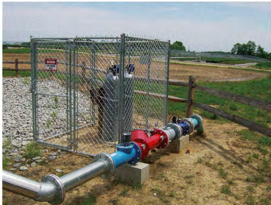
As a disinfectant, chlorine kills algae, bacteria and other organisms in the water supply. Chlorination also eliminates the energy source for iron bacteria. Chlorine gas is injected from gas cylinders, which should be kept in a locked wire cage with a roof covering to reduce potential human exposure to gas chlorine when changing cylinders.
