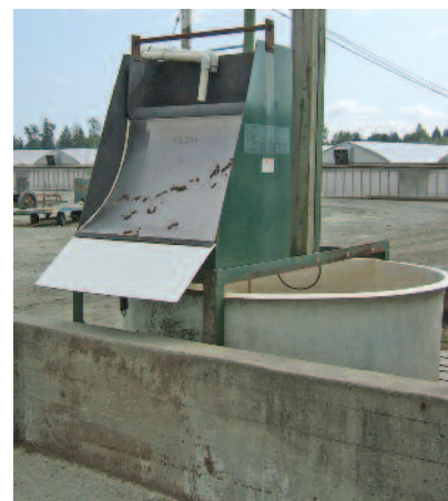
LAMINAR FILTER – PERMITS WATER REUSE IN BLOCKWASHING.
