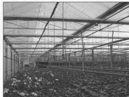
Growers considering installing energy/shade curtains should make an energy savings investment calculation for each greenhouse compartment to determine the priority for investment.
