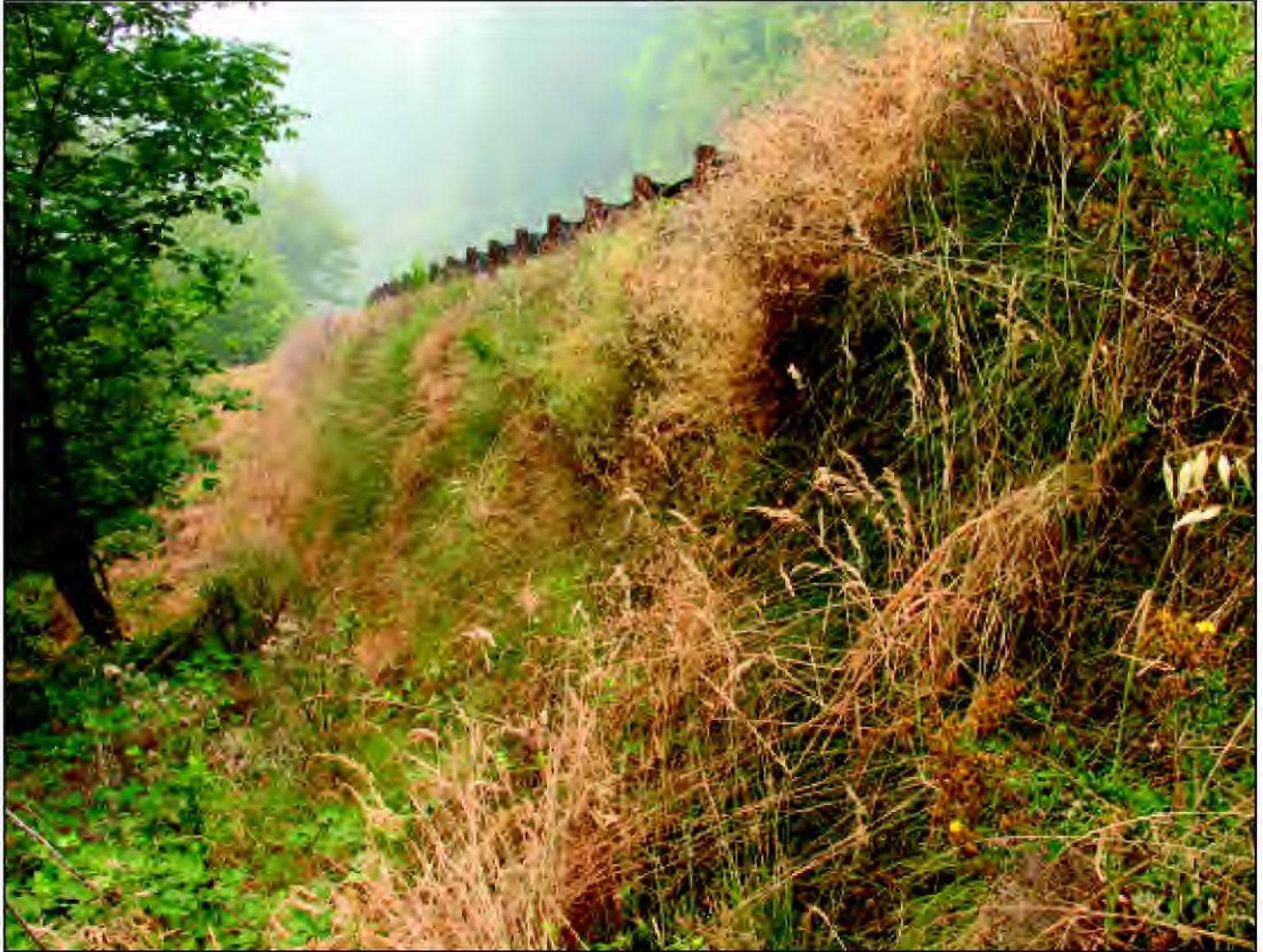
Three years after installation, native grasses are well established on 20 feet high soil faced retaining walls.
