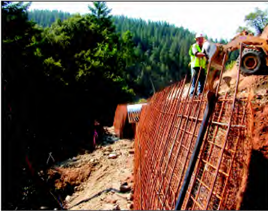
As retaining walls were built, seeded mats were attached to the frames and filled behind with a foot of topsoil.
