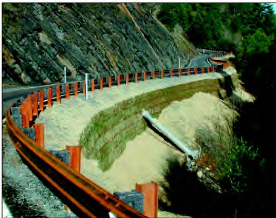
Above: 2003. Grass seeds began to germinate in late fall, three months after wall installation. Below: 2006. Three years later, retaining walls are screened by strands of native grasses.
