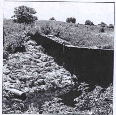
Water control structure constructed for treatment wetland project in Boone County, Iowa.
