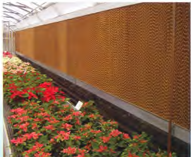
Evaporative cooling pads are installed along the inside of a greenhouse ventilation inlet opening.
